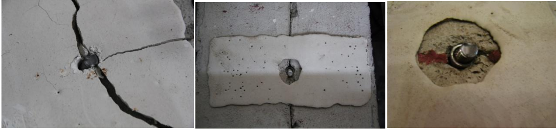
Figure 4. Failure point for three different shear test cycles. The rod failed in all three cases.
